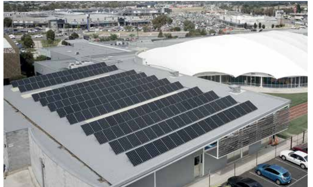
Catching rays: More than 300 solar panels were installed at Leisurelink Aquatic Centre as part of the City's Zero Carbon Buildings Program.
